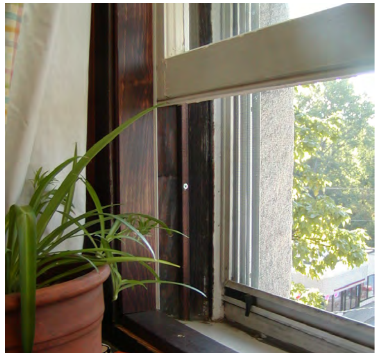
This window upgrade included truing sashes to fit the opening, adding leaf seals (see the white seal on the left, against the outside edge of the interior jamb trim), and routing in a beefy sill gasket.
